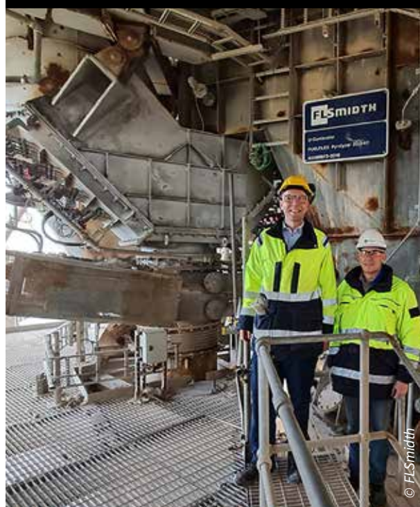
Mannok Cement and FLSmidth collaborated to install a FUELFLEX® Pyrolyzer at the producer's plant in Ireland
